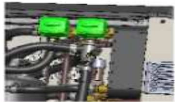
Mixing valves in series
